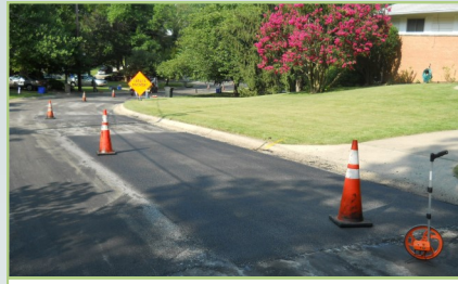
Patching may be necessary prior to resurfacing
