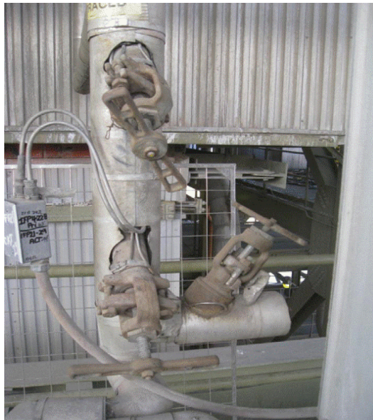
Figure 6: Exposed valves emerge from thermal insulation and are not heat traced
