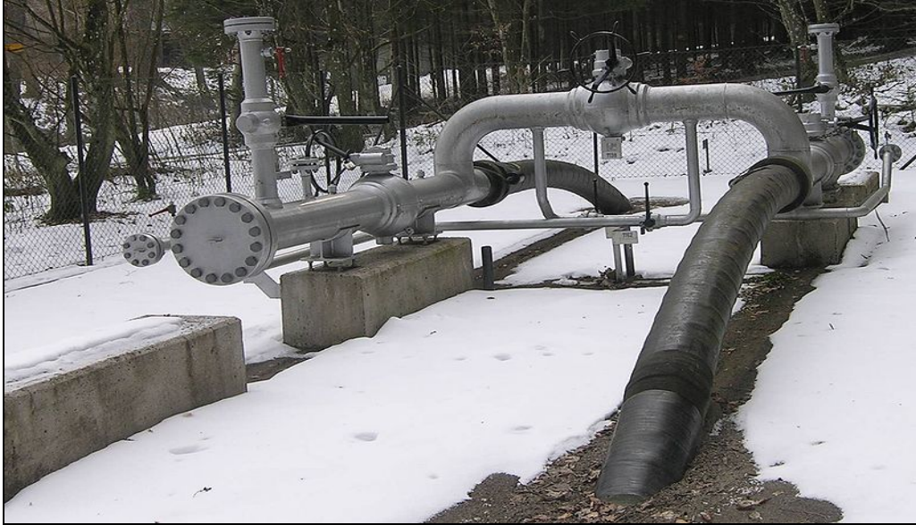
Figure 12 – Pipeline Pig Launch and Receiving Station (Photo credit Wikimedia Commons).
