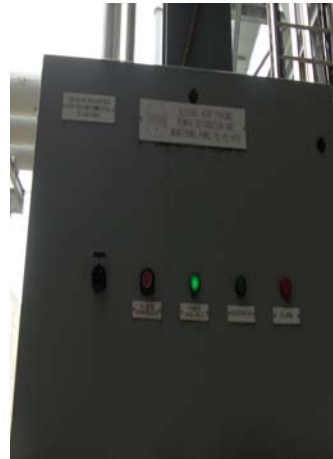
Figure 2: Freeze Protection Panel Exterior
