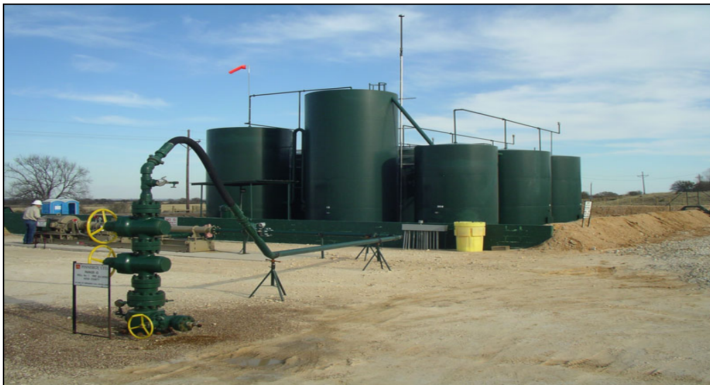
Figure 13 - Typical wellhead in Warm Climate. (GTI) No methanol or other injection equipment for freeze mitigation. Flow line is elevated without insulation of other protection from cold weather. Tank battery and other production equipment are not protected from cold weather. (Ref. 4)
