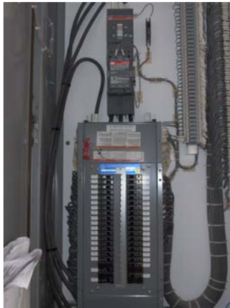
Figure 1: Freeze Protection Panel Interior
