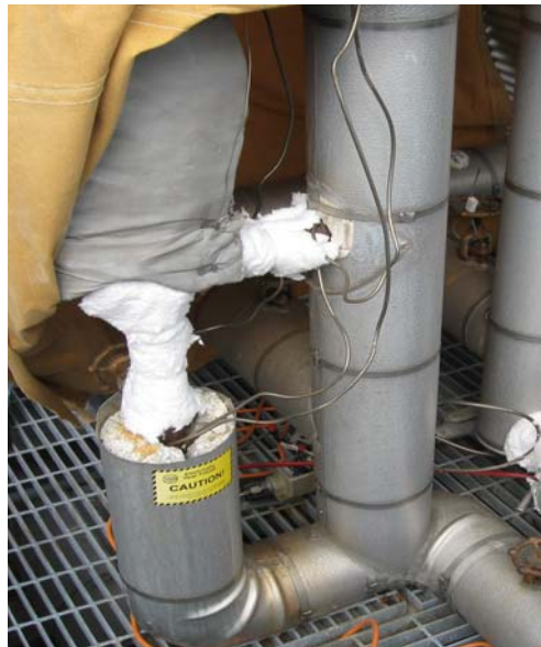
Figure 4: Insulated Piping with Heat Tracing
